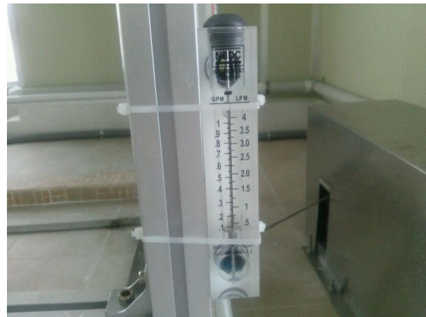
Water flow meter with Drip box
