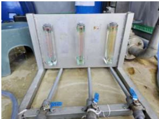
Area flow meter
