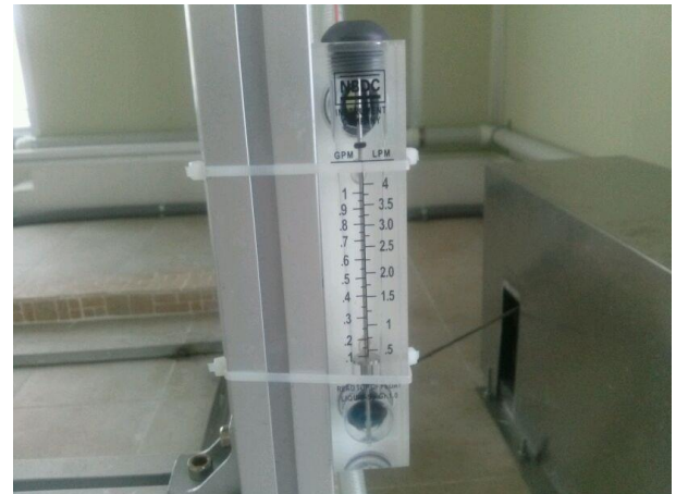
Water flow meter with Drip box
