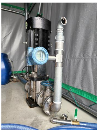
Area flow meter
