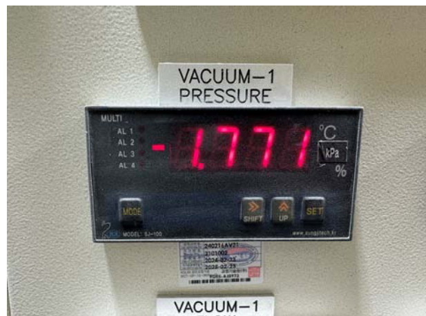
Digital vacuum pressure gauge
