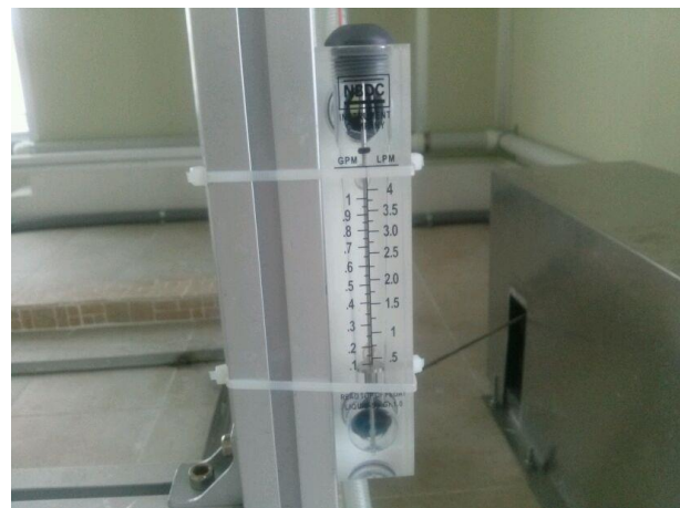
Water flow meter with Drip box
