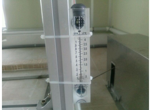
Water flow meter with Drip box
