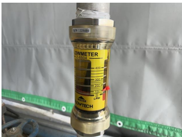
Area flow meter
