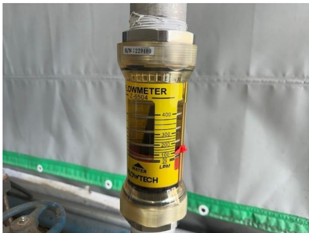
Area flow meter
