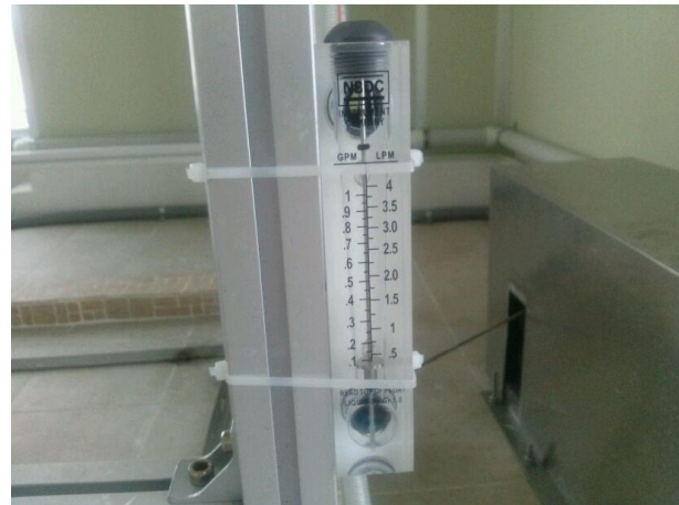
Water flow meter with Drip box
