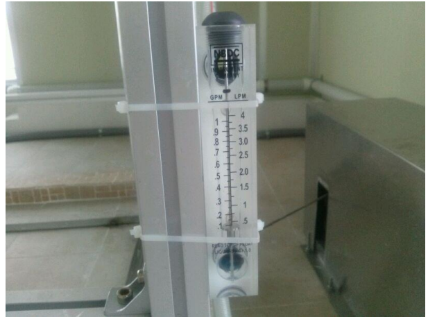
Water flow meter with Drip box
