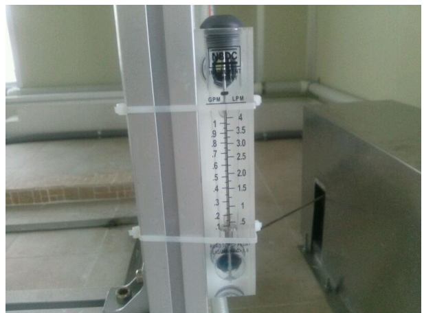
Water flow meter with Drip box
