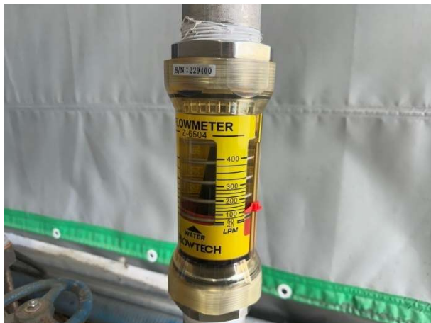
Area flow meter
