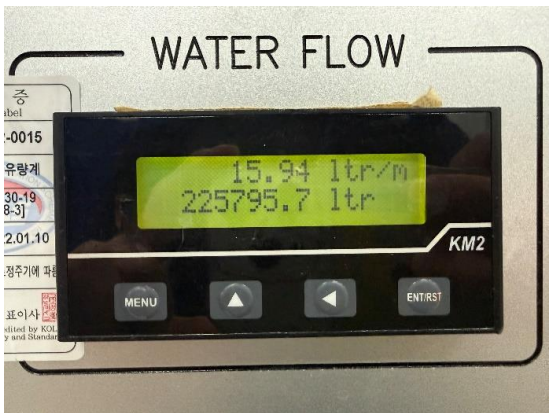
Figure 16) Photo of test condition (flow rate)
