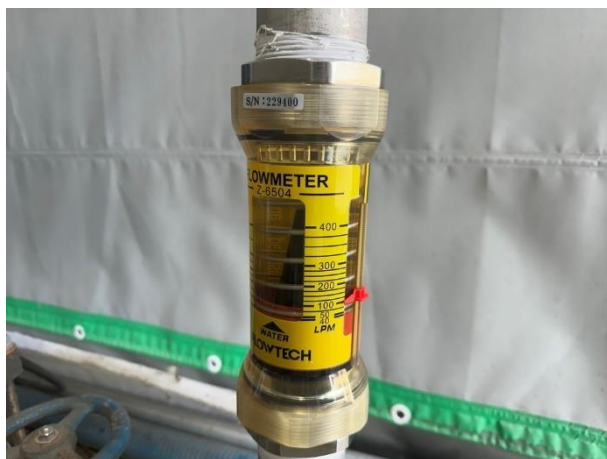
Area flow meter
